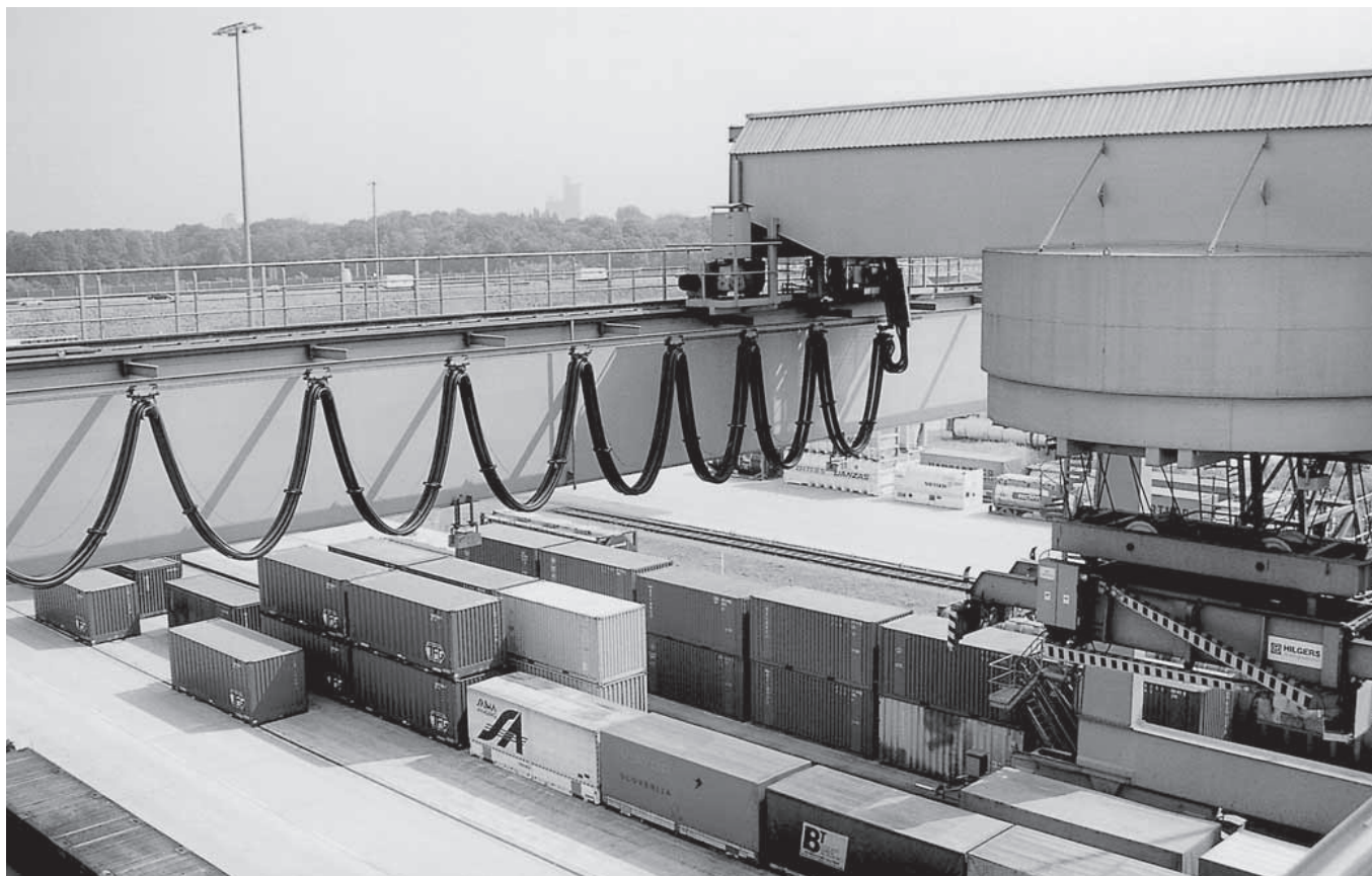
Cable carrier at a container crane
